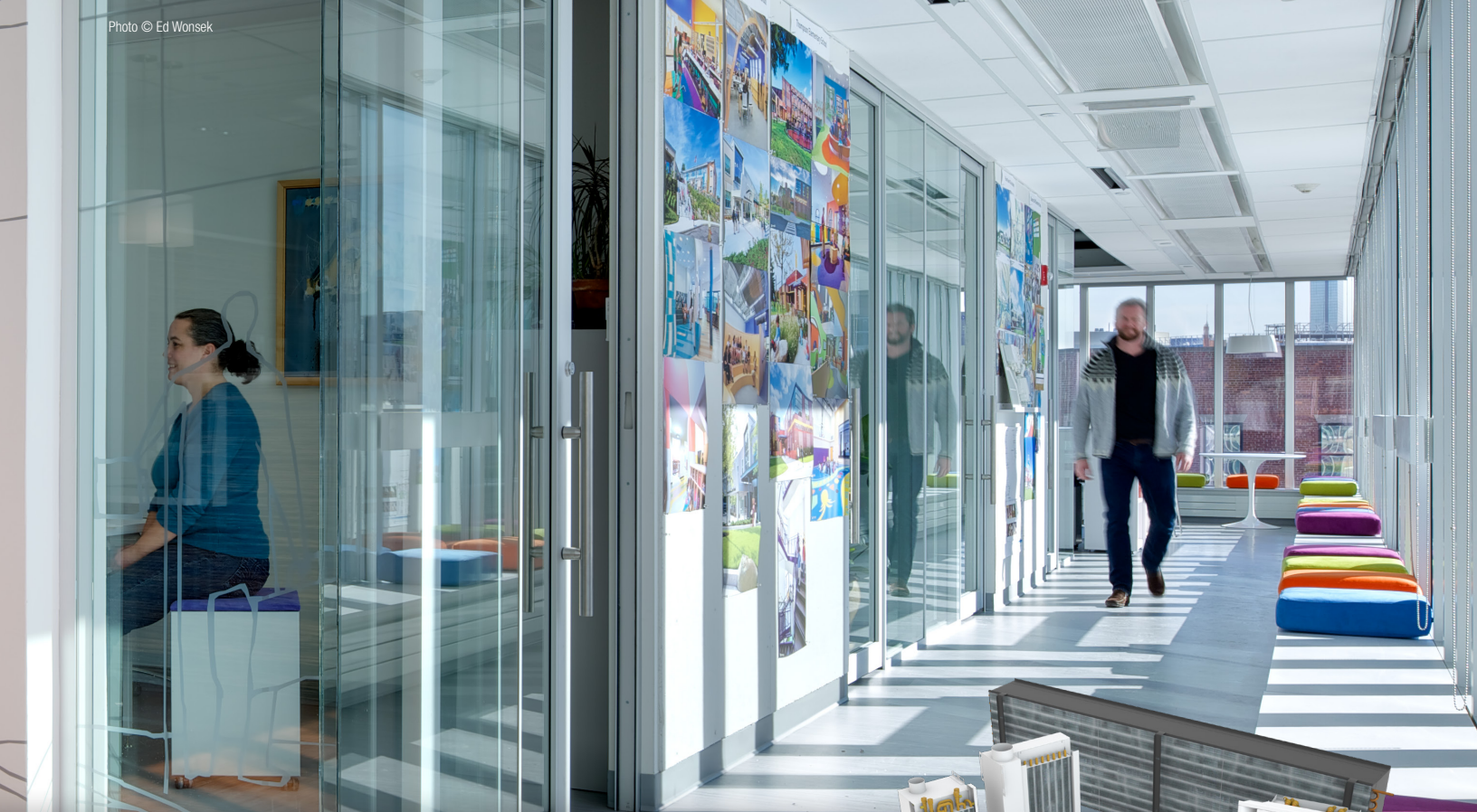
Above: Chilled Beams
